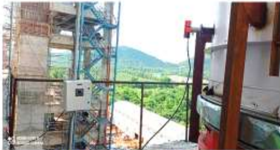
PM Analyzer at Cement Mill Stack
