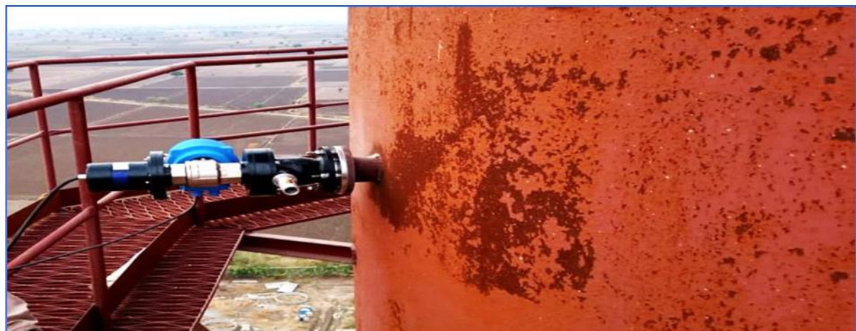
PM CEMS for Clinker Cooler ESP Stack
