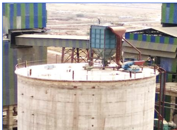
Bag Filter at Flyash Silo top
