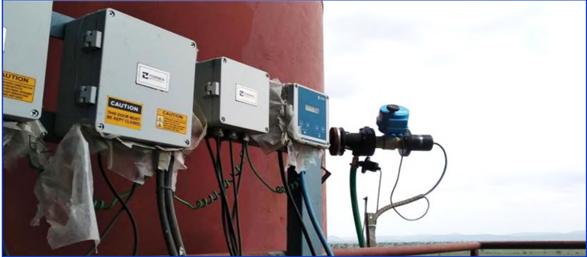
PM CEMS for Cement Mill Bag House Stack
