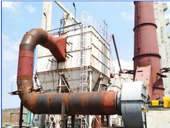
Bag Filter for Crusher
