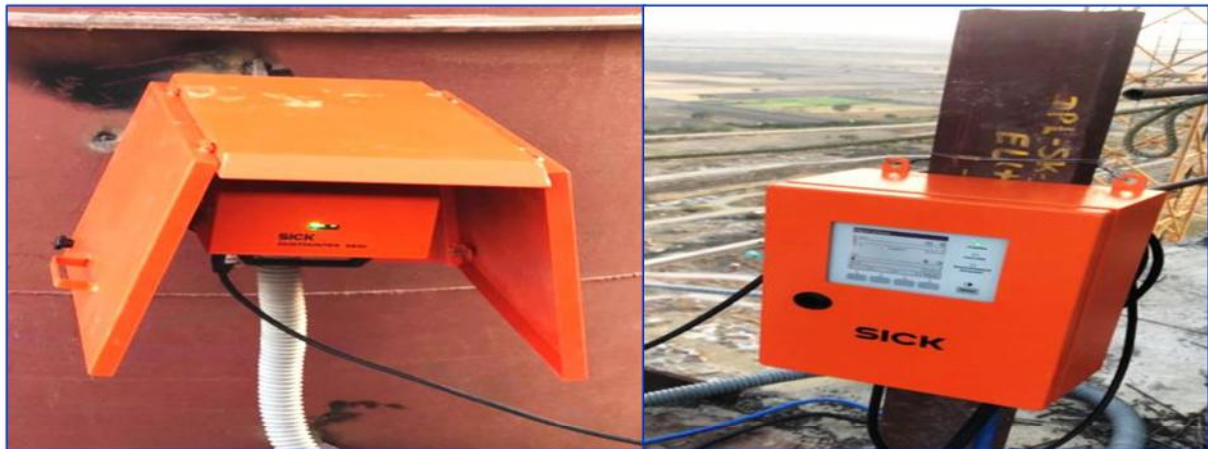
PM CEMS for Coal Mill Bag House Stack
